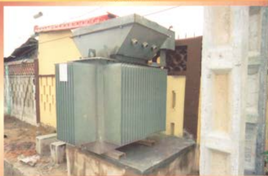
One of the installed transformers by the Hon. Adekanye-led administration
