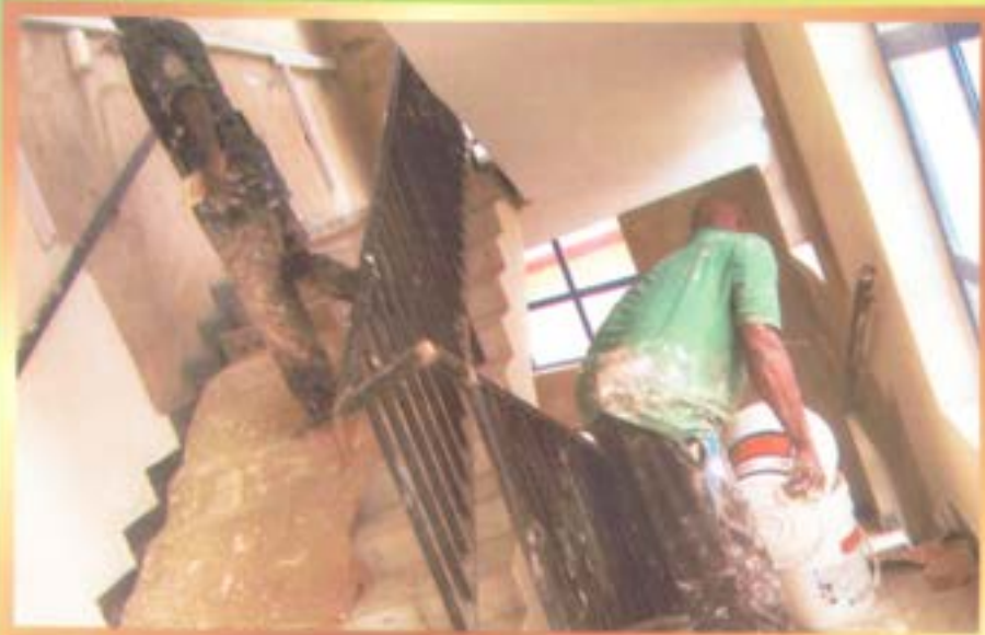
Wall pop of the newly constructed secretariat building in progress
