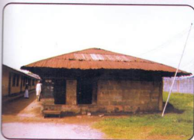
Certified structurally defective classroom block
