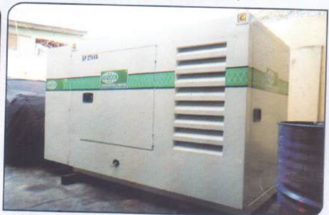
Newly purchased Generator for Oloto's Palace by LMLG & Yaba LCDA
